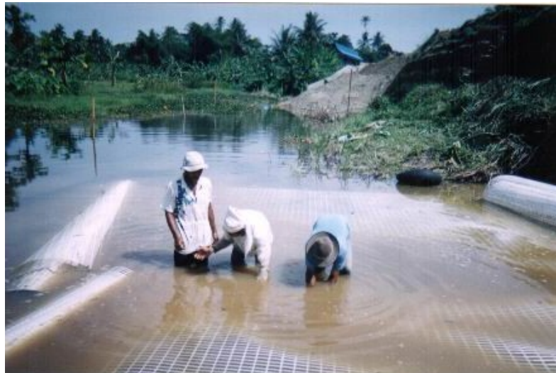
Figure 13. Extreme soil conditions on site
