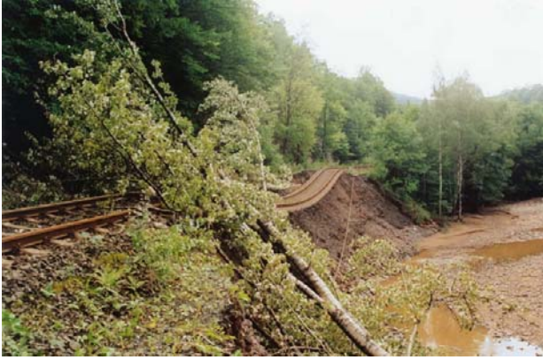
Figure 18. Collapsed railway embankment after flooding
